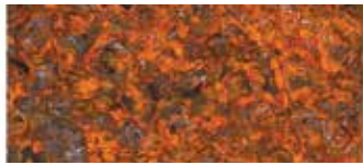
Without corrosion protection treatment
